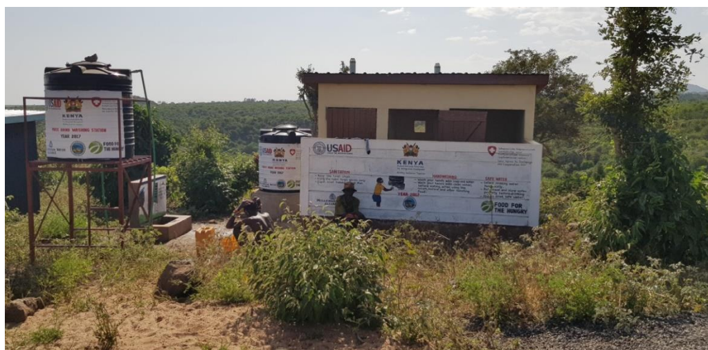
A raised hand washing tank and rain water harvesting tank at Ilpus Primary School, Marsabit County constructed through Kenya RAPID support. Photo credit: Johnson Ng’ang’a.
