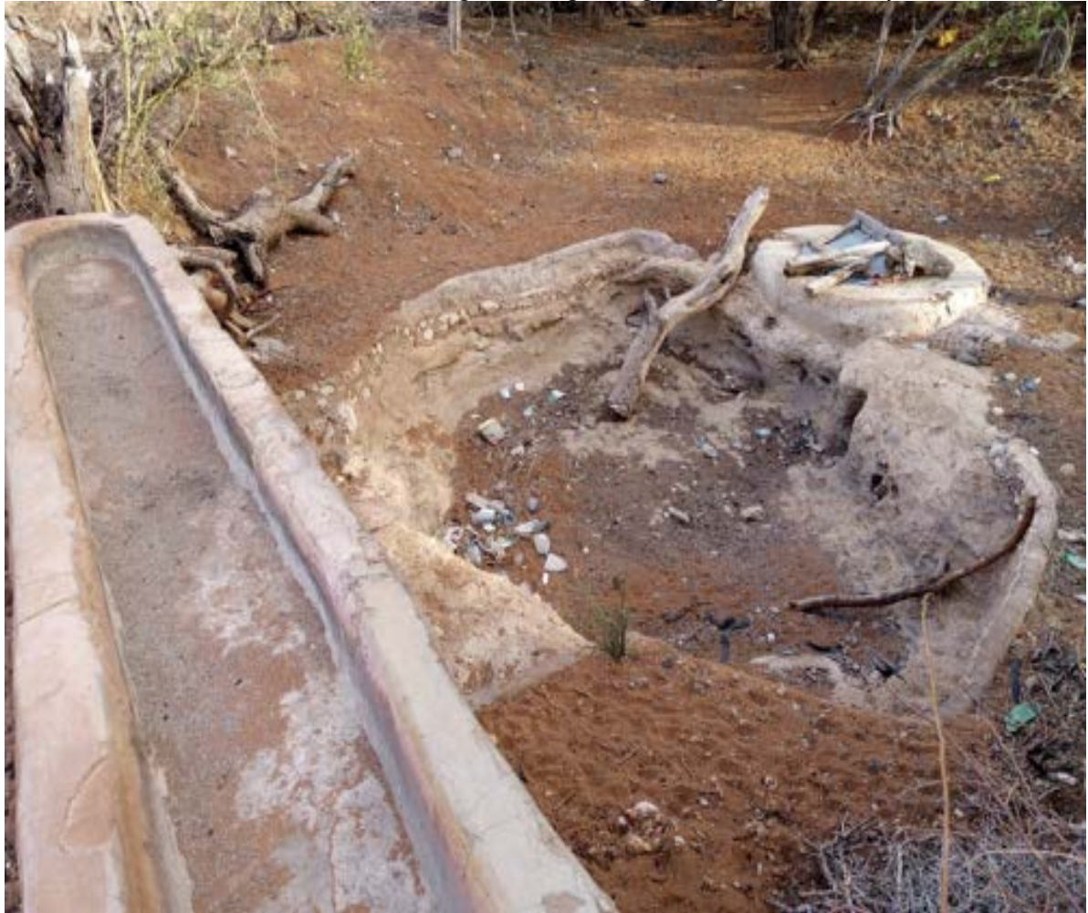
Abandoned water trough at Ndugu Zangu village, Isiolo County
